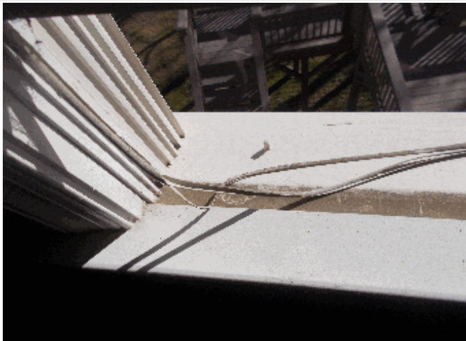
Interior: Loose bottom seals on back upper bedroom window(s)
