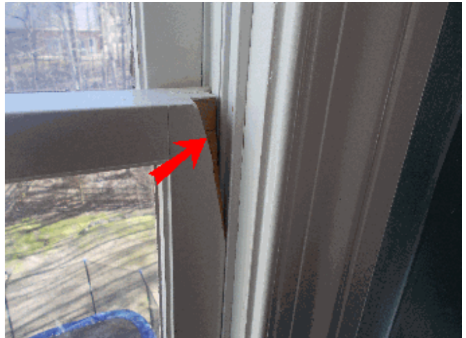
Interior: Piece of window sash is broken - back upper bedroom
