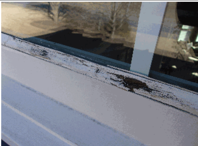
Structure: Rot on arch window above the front entrance
