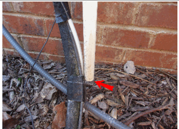
Heat: We recommend extending the HVAC condensation lines away from the house
