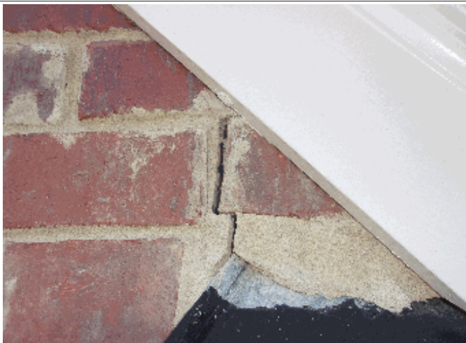
Exterior: Crack above the porch roof should be sealed
