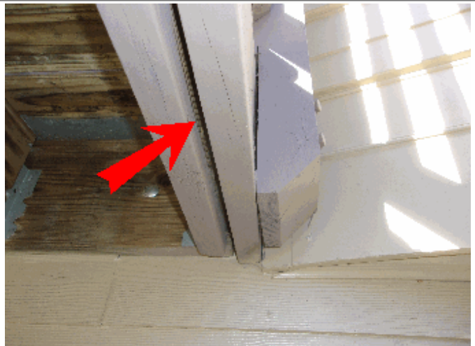
Exterior: Deck band pulled way from joists near bay - lag bolts do not appear to have pierced the joist
