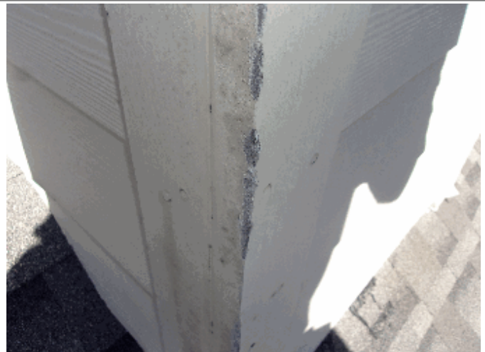
Exterior: Some of the trim on the chimney needs to be painted
