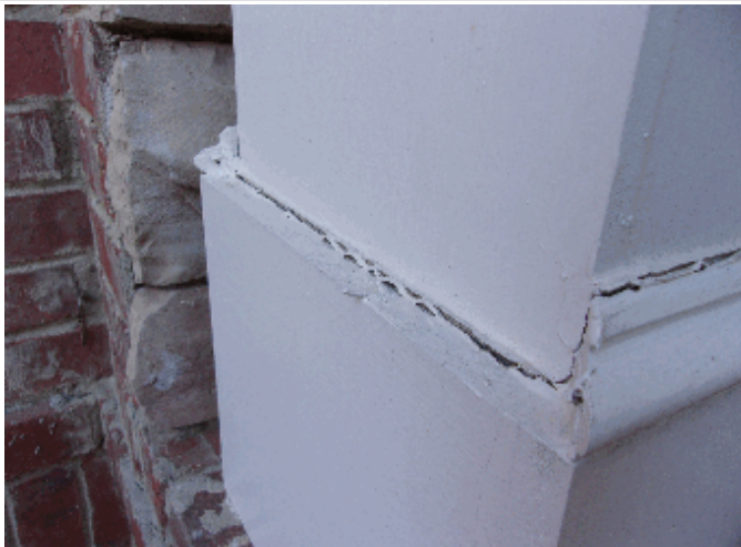
Trim is missing on front porch column and it needs to be caulked
