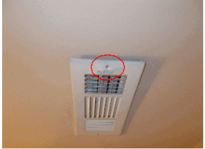
Heat: Screw missing on vent cover in the upstairs middle bathroom
