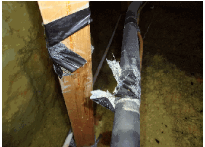
Heat: HVAC line set should be secured - attic
