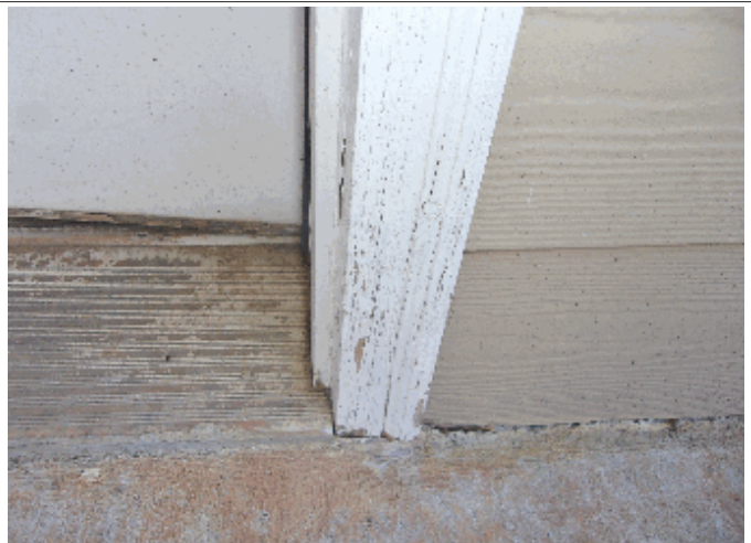
Exterior: Trim on several doors/windows need to be painted
