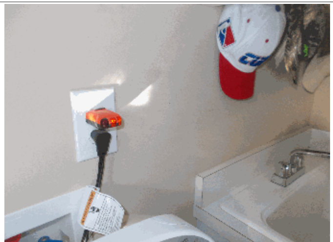
Electric: Outlet near the laundry sink is not GFCI protected
