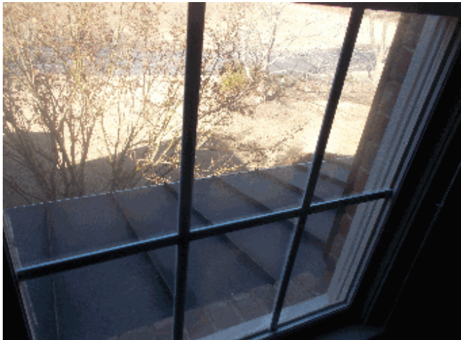
Interior: Window above the front entrance is slightly fogged
