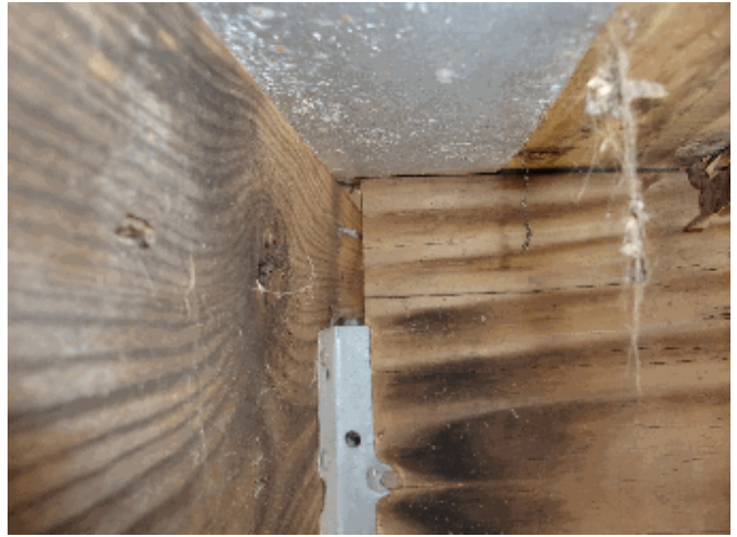
Exterior: Some deck joists are pulling away from the band - you may want to install a different type hanger
