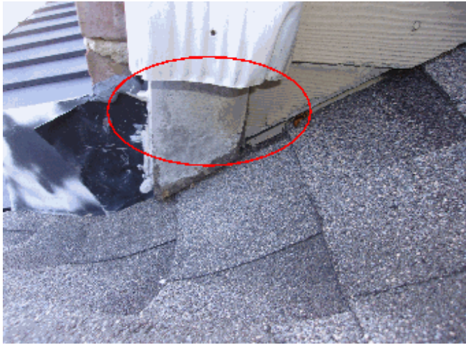
Exterior: Downspout above the roof in front needs an elbow
