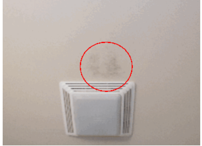
Interior: Stain on ceiling in the main floor bath appears to be from condensation
