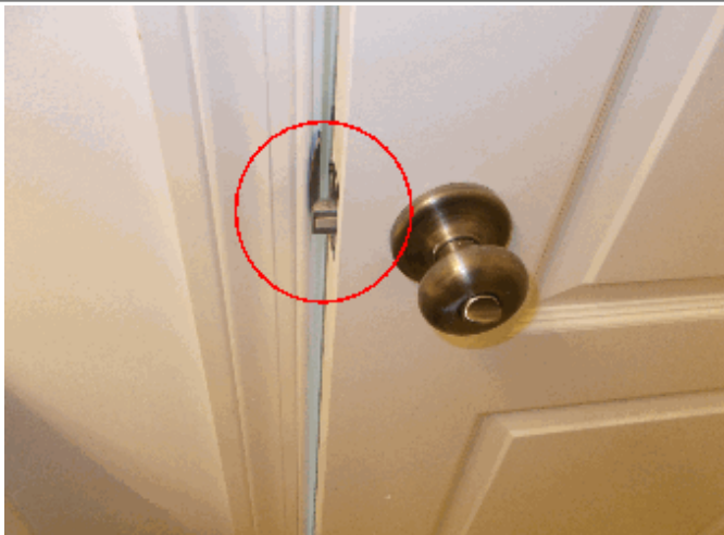
Interior: Two doors in the Jack and Jill bath would not latch
