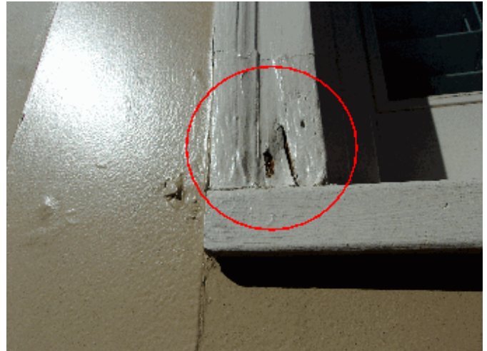
Structure: Trim rot on middle back bay window
