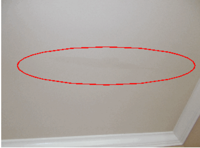
Interior: There are faint stains on the dining room and back left bedroom ceilings - no moisture reading
