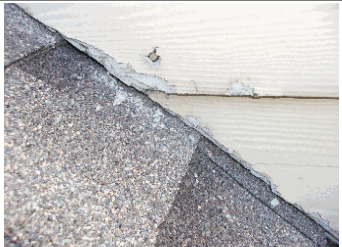
Exterior: Deteriorated siding above the roof
