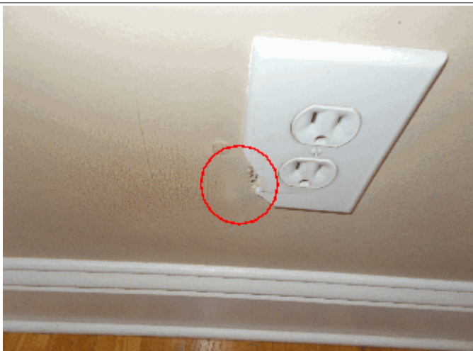
Electric: Broken cover on outlet in the foyer
