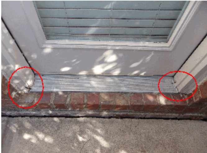
Structure: Rot on the garage man door jamb
