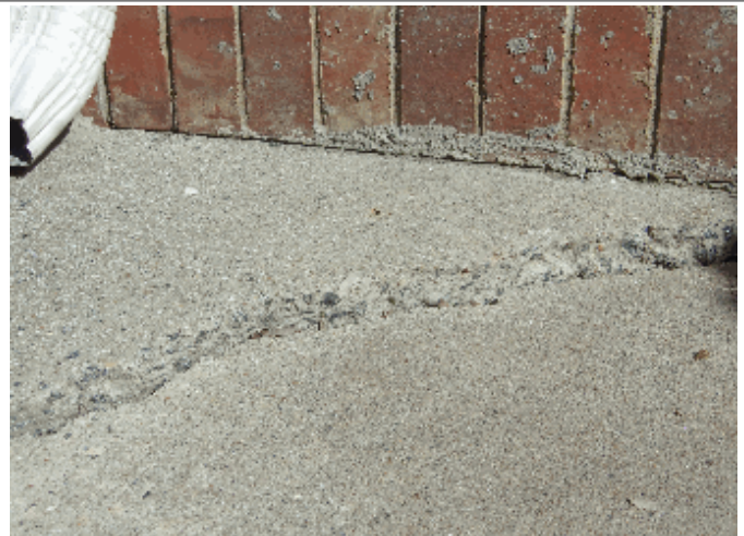
Exterior: Walkway on the right side of the house has settled; this could be a trip hazard
