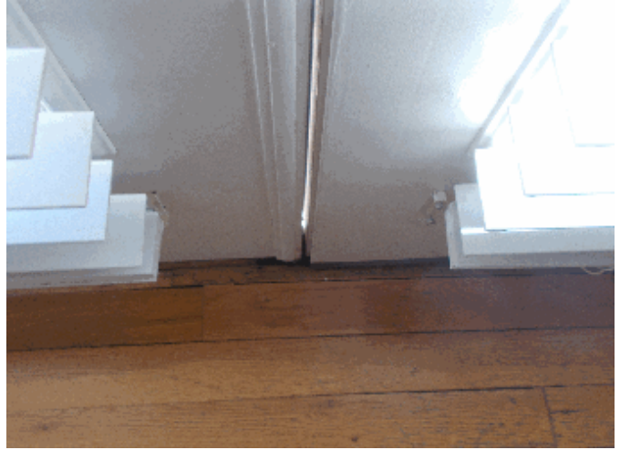
Interior: Daylight showing through back deck doors and the door is difficult to open/shut
