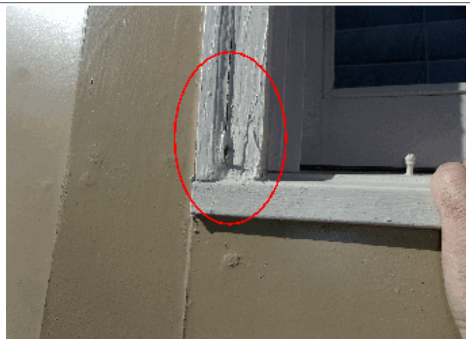
Structure: Trim rot on back left window
