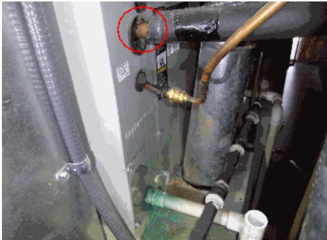
Heat: Line set should be insulated/sealed at the unit to prevent condensation - basement
