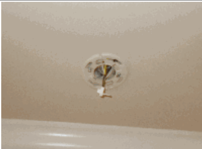
Interior: Smoke detector in the upstairs hallway has been removed
