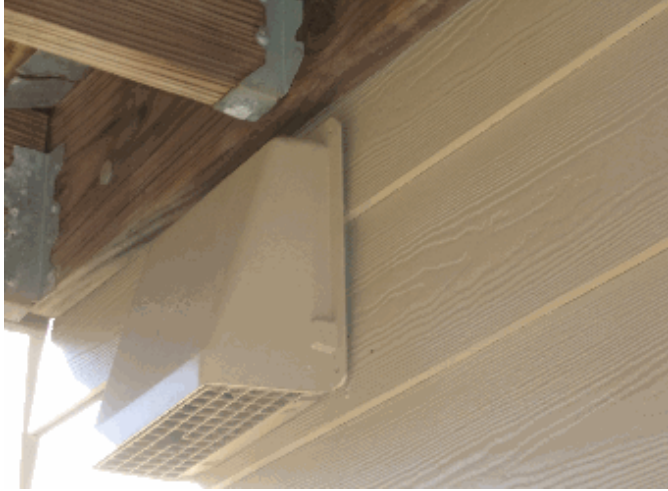
Exterior: We recommend sealing around all vents on the outside and cleaning the dryer vent prior to use
