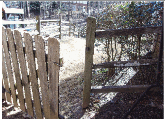
Exterior: Fence gate on the left does not open/shut properly
