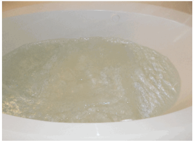
Jetted tub operated in the master bath
