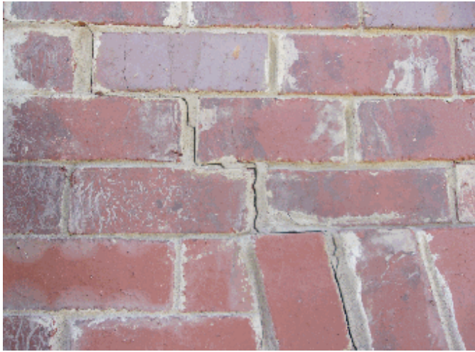
Exterior: Cracks in brick above the garage
