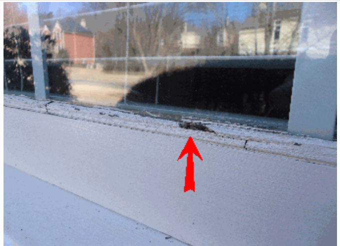
Rotted window sash on lower left front window; other windows have some rot as well
