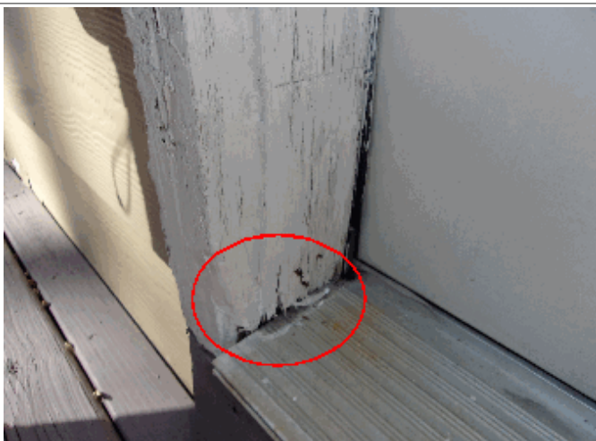
Structure: Rotted trim on the back deck door
