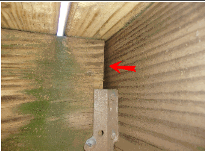
Exterior: Some joists are pulling away from the outside deck band
