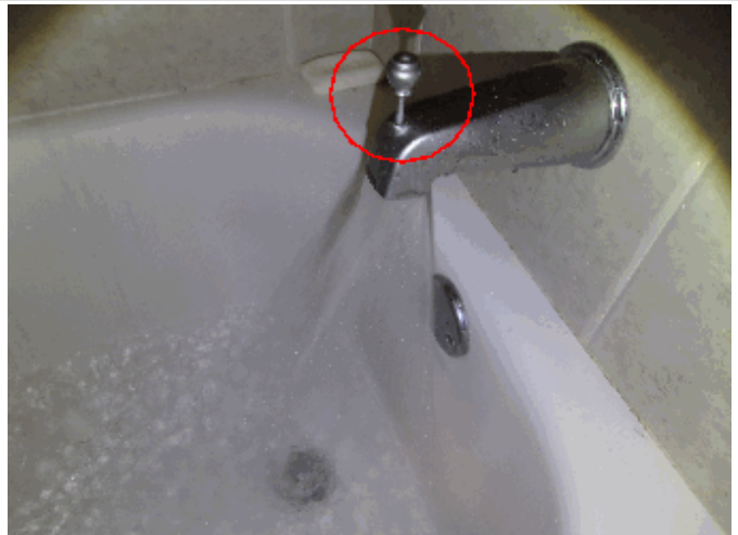
Shower diverter would not close completely in the basement bath
