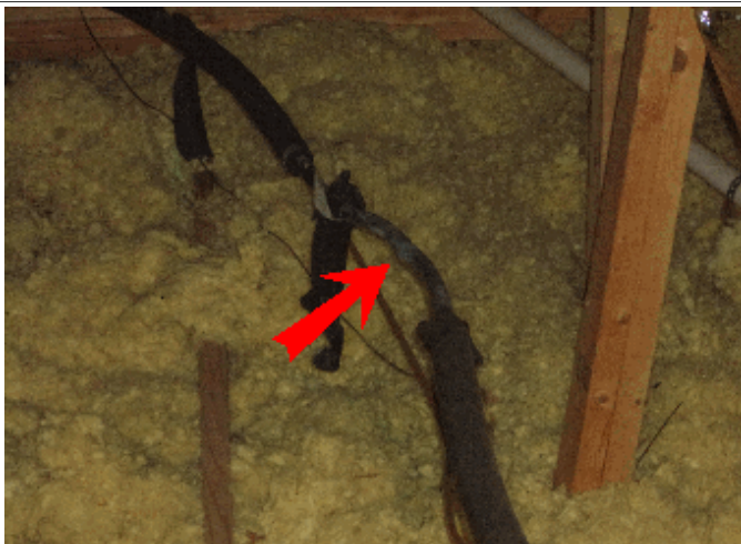
Heat: Section of the line set above the closet in the left upper front bedroom condensates causing ceiling stain
