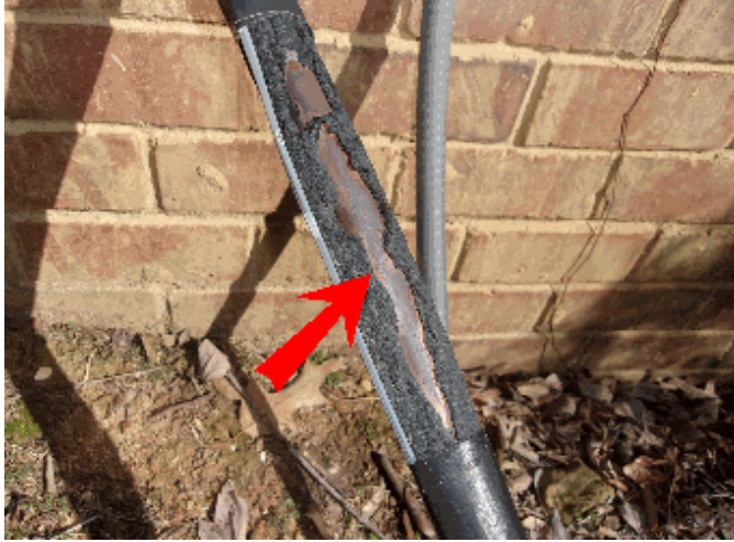
Heat: Line set for the A/C unit on the right should be reinsulated
