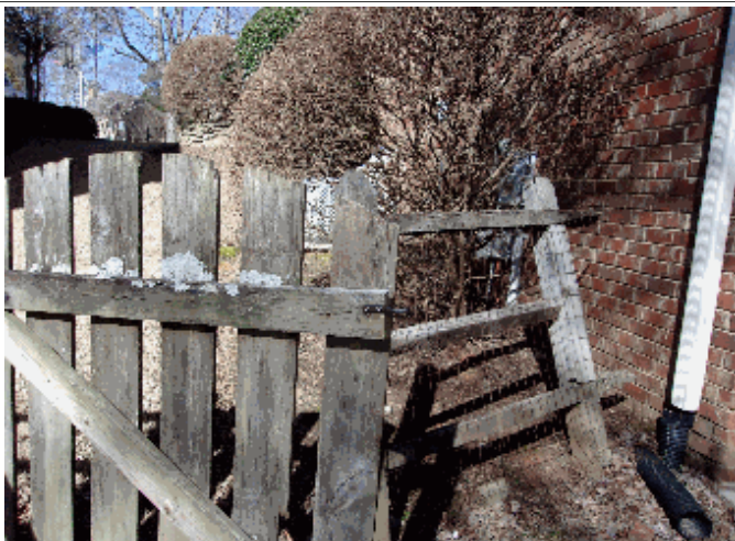
Exterior: Fence gate on the right does not open/shut properly and the posts are rotted
