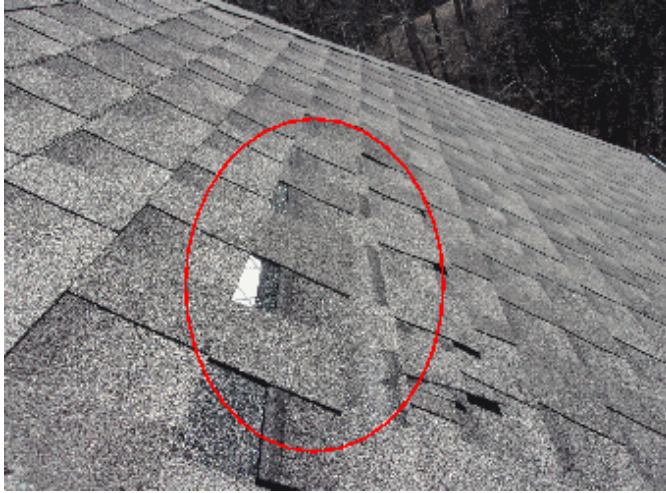
Exterior: Row of shingles on the front needs to be reattached; this will cause a leak
