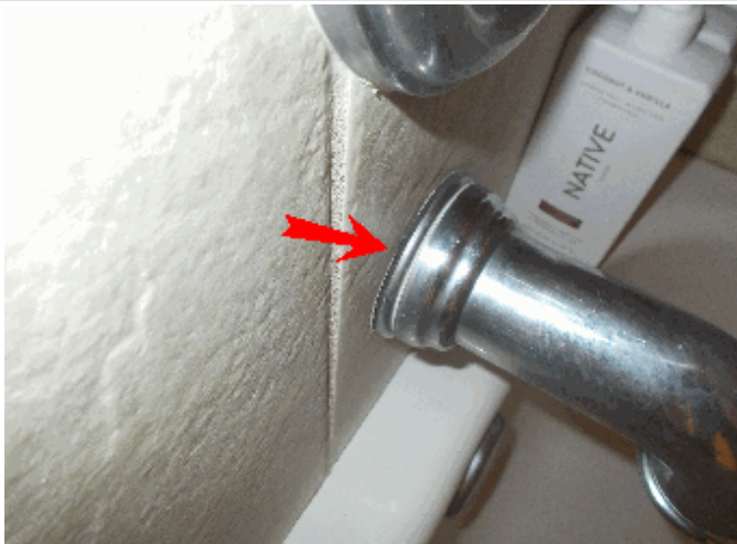
We recommend caulking around the tub spigot in the Jack and Jill bath
