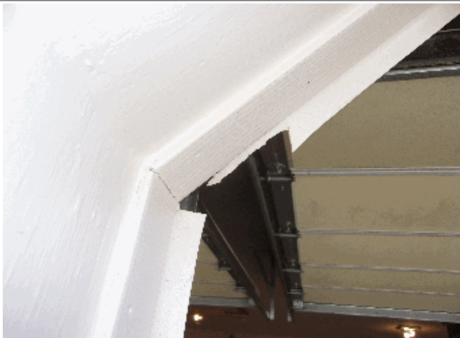
Exterior: Minor damage to garage door seal
