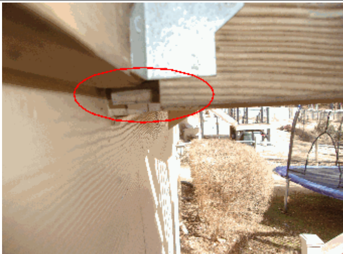
Exterior: Some deck joists have dropped down slightly
