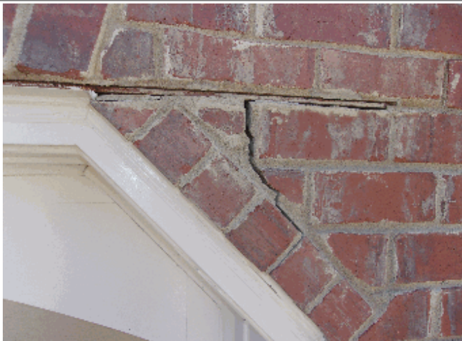
Exterior: Loose brick above the right side of the garage should be secured and sealed
