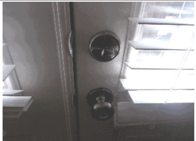
Interior: Basement double door is difficult to open/shut
