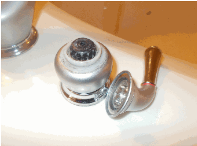
Faucet handle is loose on the master tub
