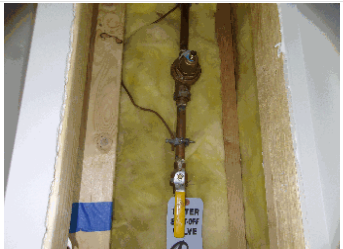
Main water shut off and pressure regulator in the basement
