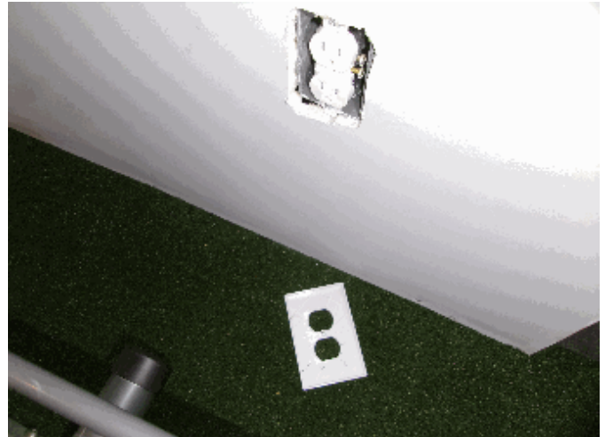
Electric: Receptacle in the basement is loose and needs the cover installed
