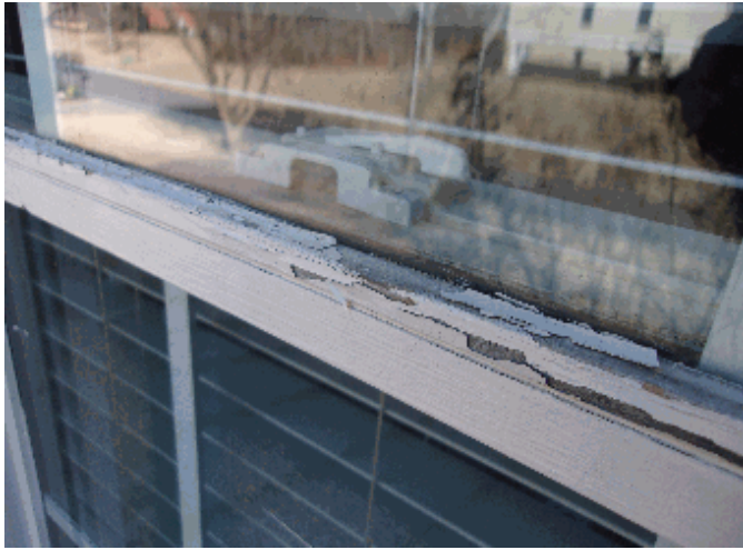
Exterior: Several windows need to be painted
