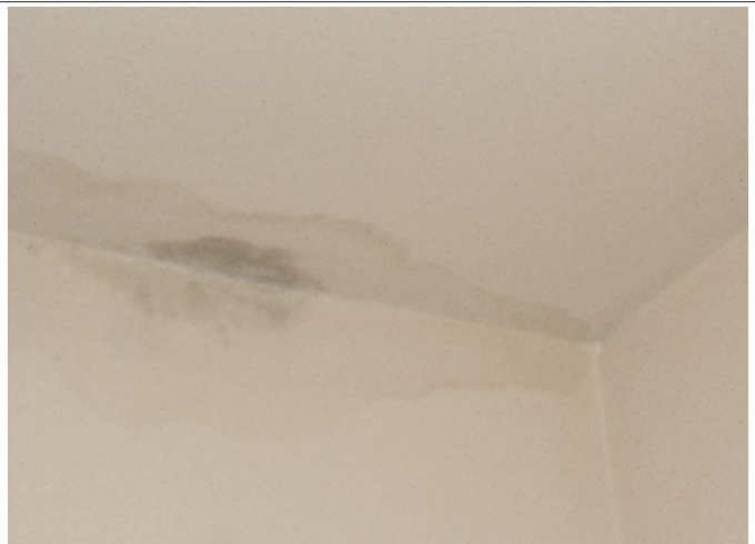
Interior: Stain in closet (upper front left bedroom) appears to be under line set that needs insulation
