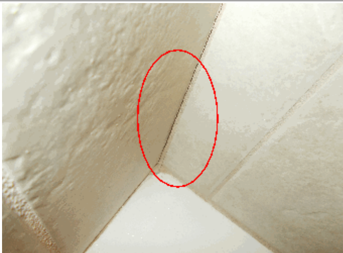
Baths1>2: You may want to seal the small cracks in the shower tile grout at some point
