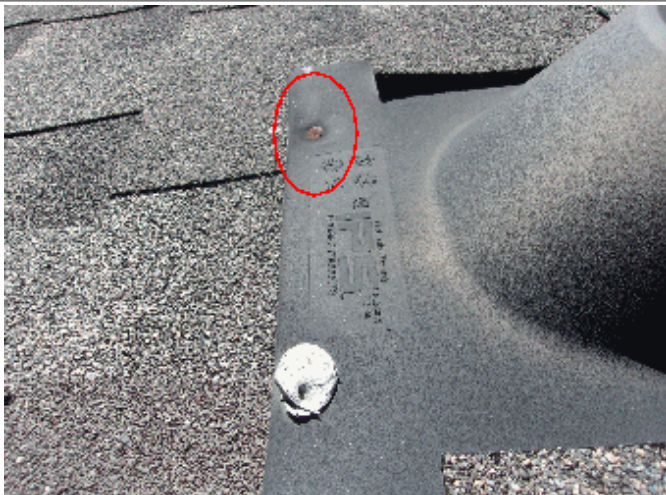
Exterior: Nail heads on vent boots should be sealed
