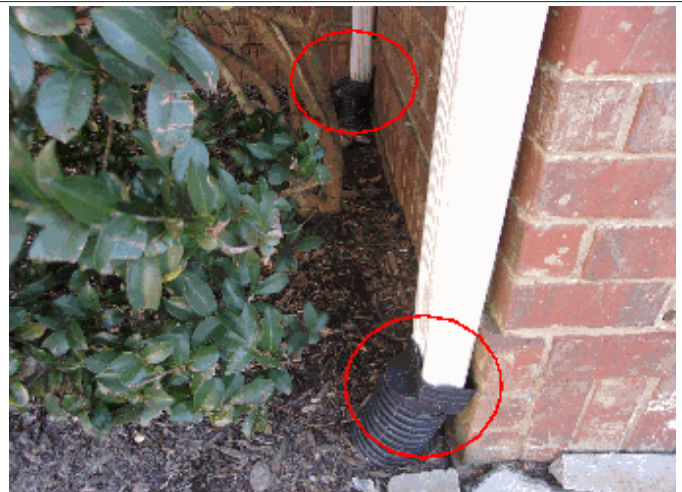
Exterior: Ensure that the two downspouts to the right of the front entrance drain properly
