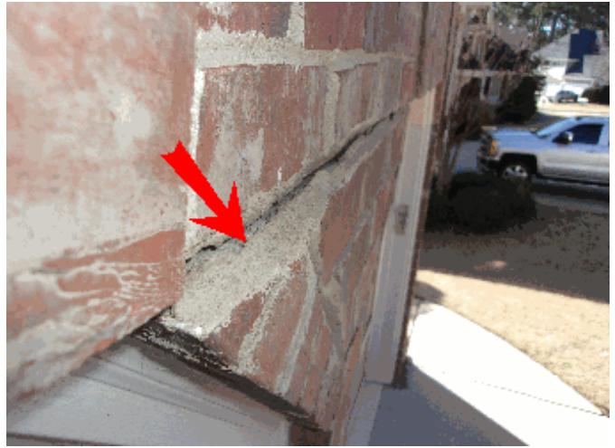
Exterior: Loose/offset brick above the garage
