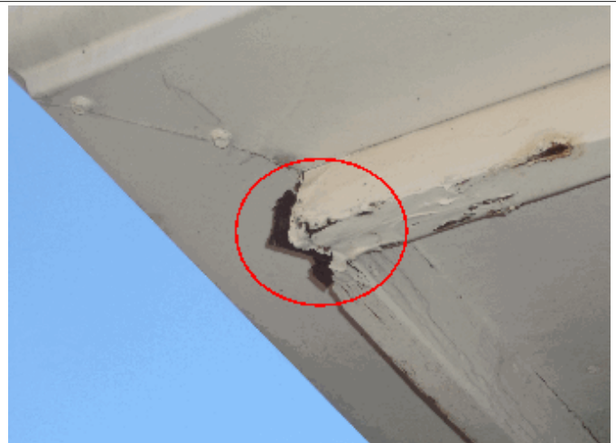
Structure: Fascia/soffit rot above the front porch
