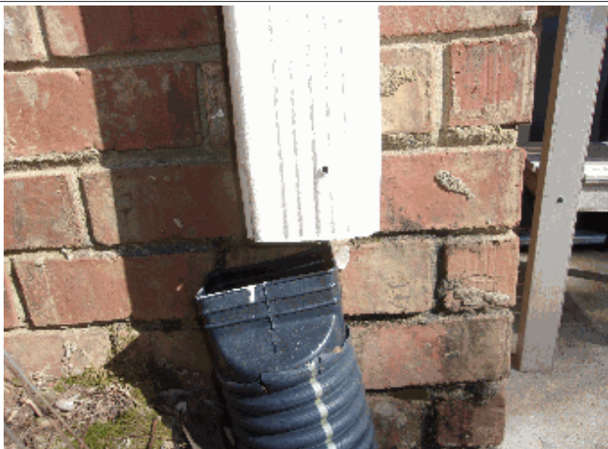
Exterior: Downspout on back right corner needs to be reattached to extension
