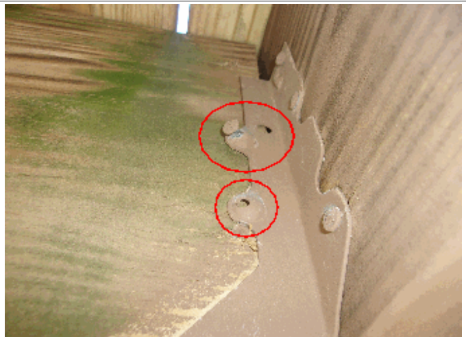
Exterior: Some of the nails on the deck joist hangers are missing and/or pulled away
